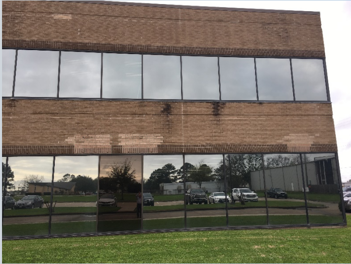
Mismatched brick and window panels
