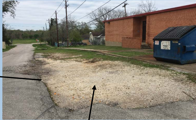
Uneven surface constricts drainage
