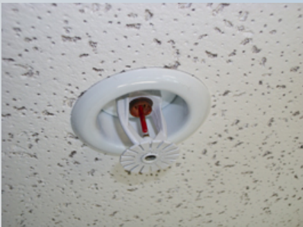
Typical Sprinkler Head
